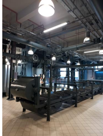
Old Heat Power Station and Power Plant. 🌟
